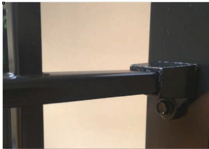
Figure 10 – Example of an Installed Iron Fence Bracket with Self-Tapping Screw
